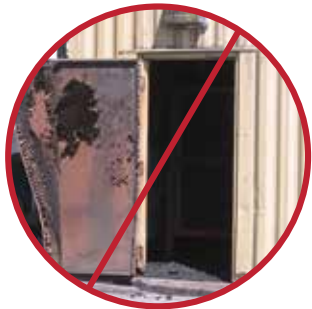
Failed Hollow Metal Door
