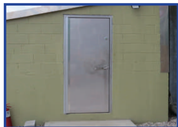
Mechanical Room Flood Door (PD-525)
